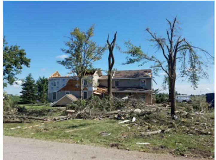
The Allen County tornado damaged this home near the intersection of Doehrman and Ehle roads. (NWS photo)
